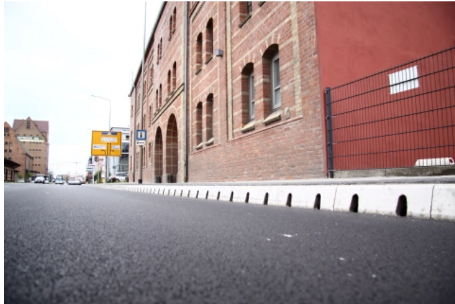
Landstraße L 22 Rostock – ACO DRAIN® KerbDrain City
