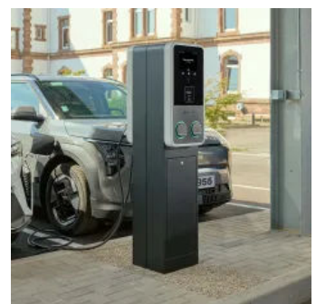
Ladestation witty park 2
